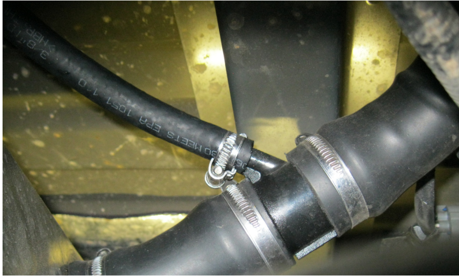
Figure 12. Transfer Flow fuel tee installed in the main fuel filler hose.
