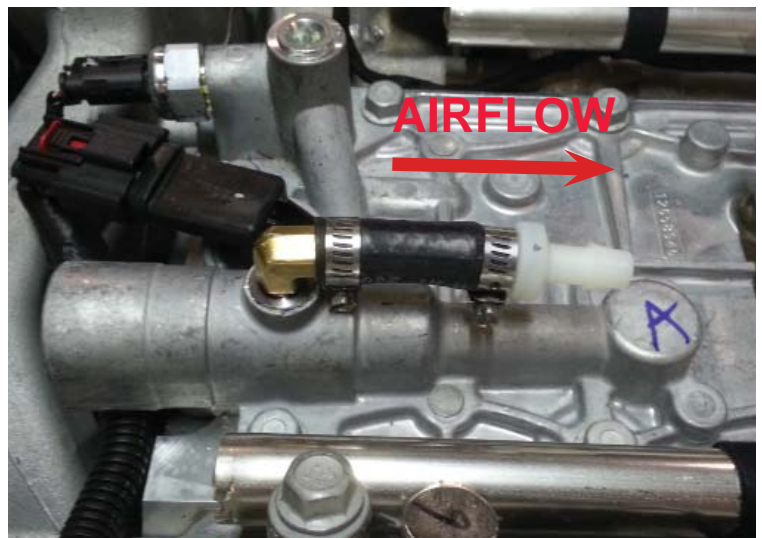
Check Valve Installed
