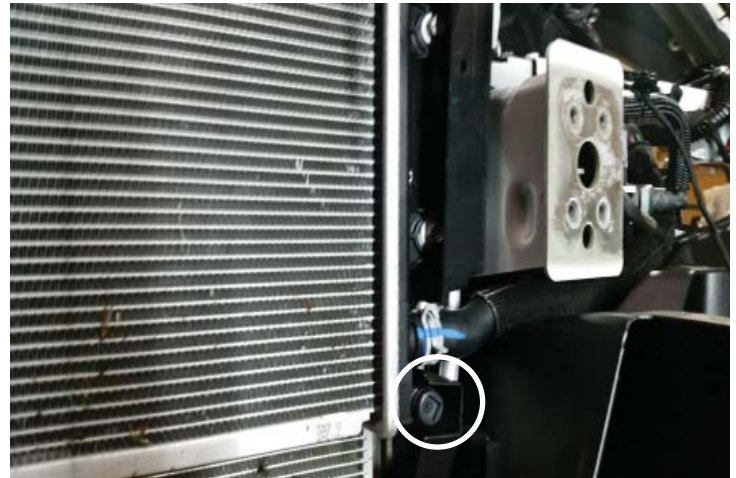
Heat Exchanger Drain
